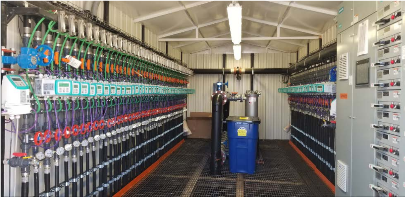
Figure 1: Inside of Header House 2 from Mine Unit 2 at URE's Lost Creek ISR plant in Wyoming. Roughly 2:1 ratio of Injection to Recovery wells.
