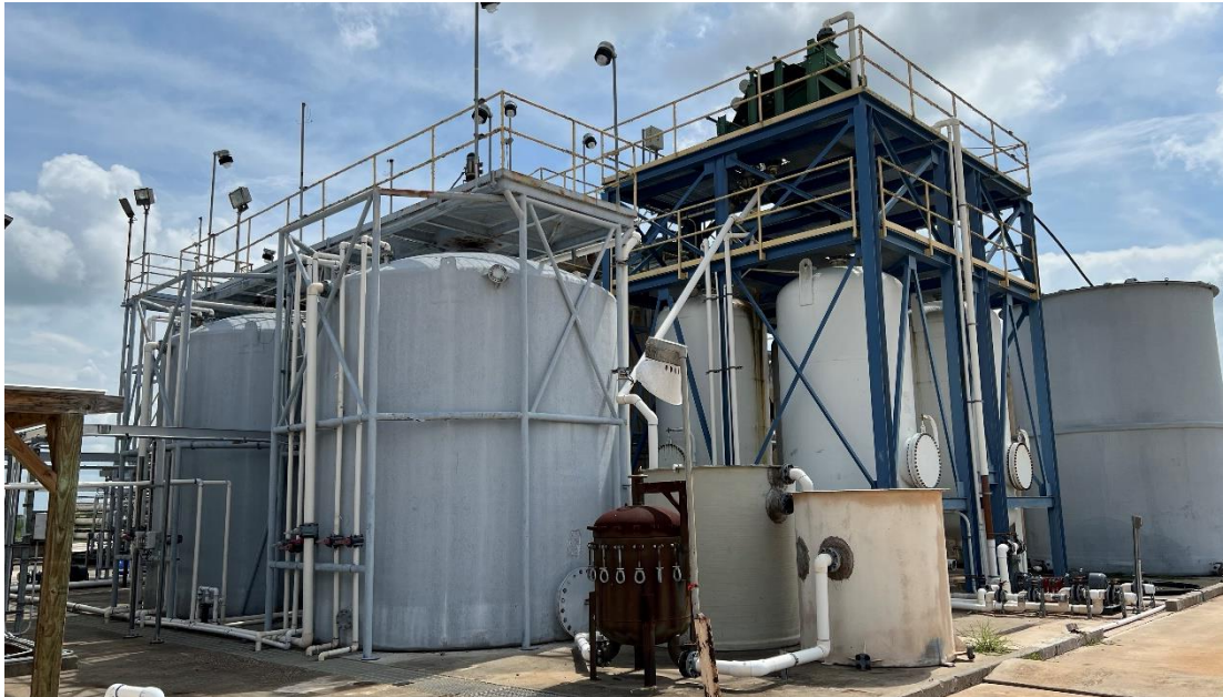
Figure 4: Rosita Plant - Fluid handling circuits - Elution, Precipitation (upper), Filtration (middle) Reverse Osmosis Treatment System and (lower) – filtration and RO systems are located behind tanks in upper picture)
