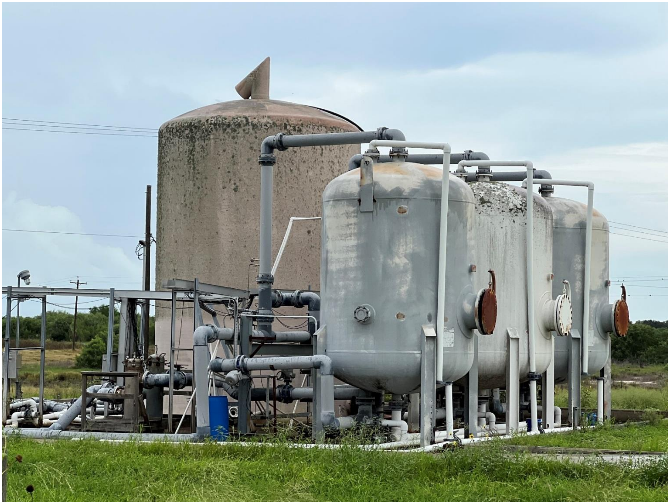
Figure 18: Kingsville Dome - example of a satellite facility available to be relocated to Rosita Extension or USC
