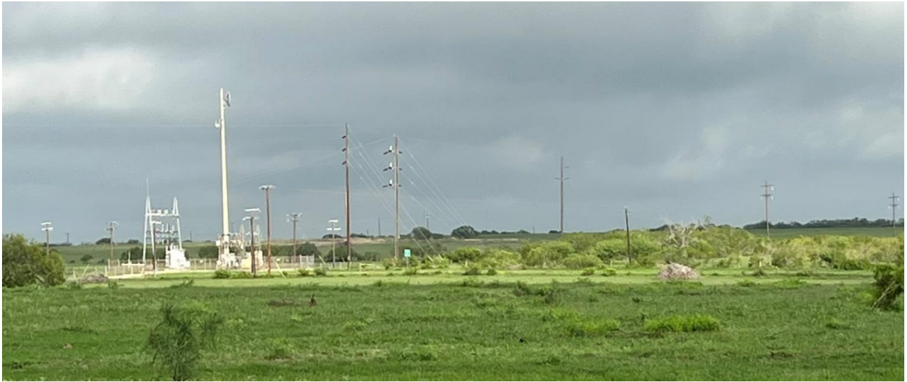
Figure 13: Upper: Significant power infrastructure in place at USC installed during prior operations. Lower: Drill rigs turning at Geffert
