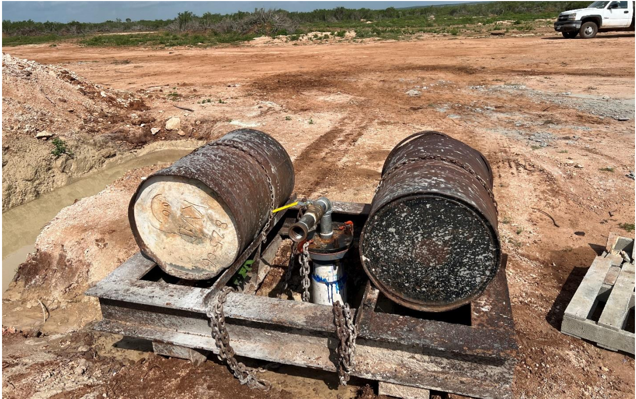
Figure 11: Rosita Extension cased production well utilizing weights to prevent ejection during concrete injection and cure (top) - Bottom (left to Right) – 1) Preparation for Mechanical Integrity Test of new well (logging truck also present), 2) Drilling new well
