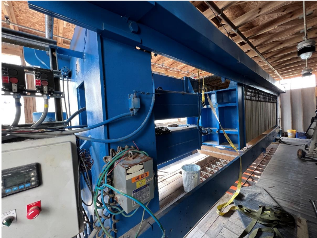
Figure 5: Rosita Plant Filter Press (upper), Drier (lower left) and Steam Generator for Drier (lower right)
