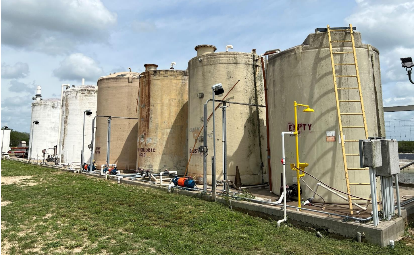
Figure 6: Rosita Plant Reagent Storage (right side, upper) & Treated water holding (left side upper), Holding Ponds (lower)
