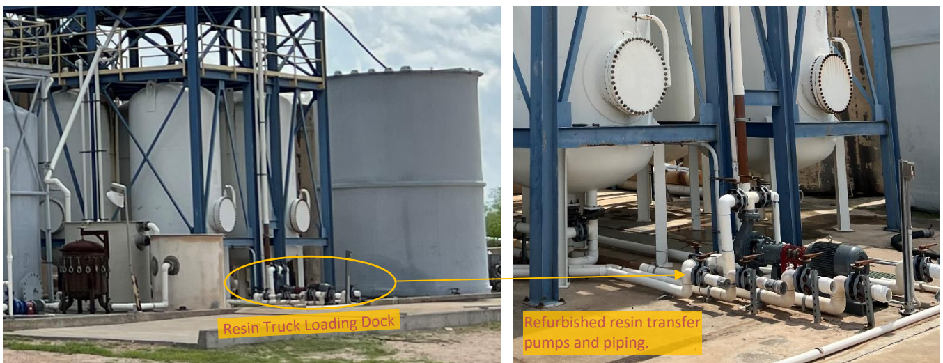
Figure 3: Rosita Plant Resin loading / unloading dock
