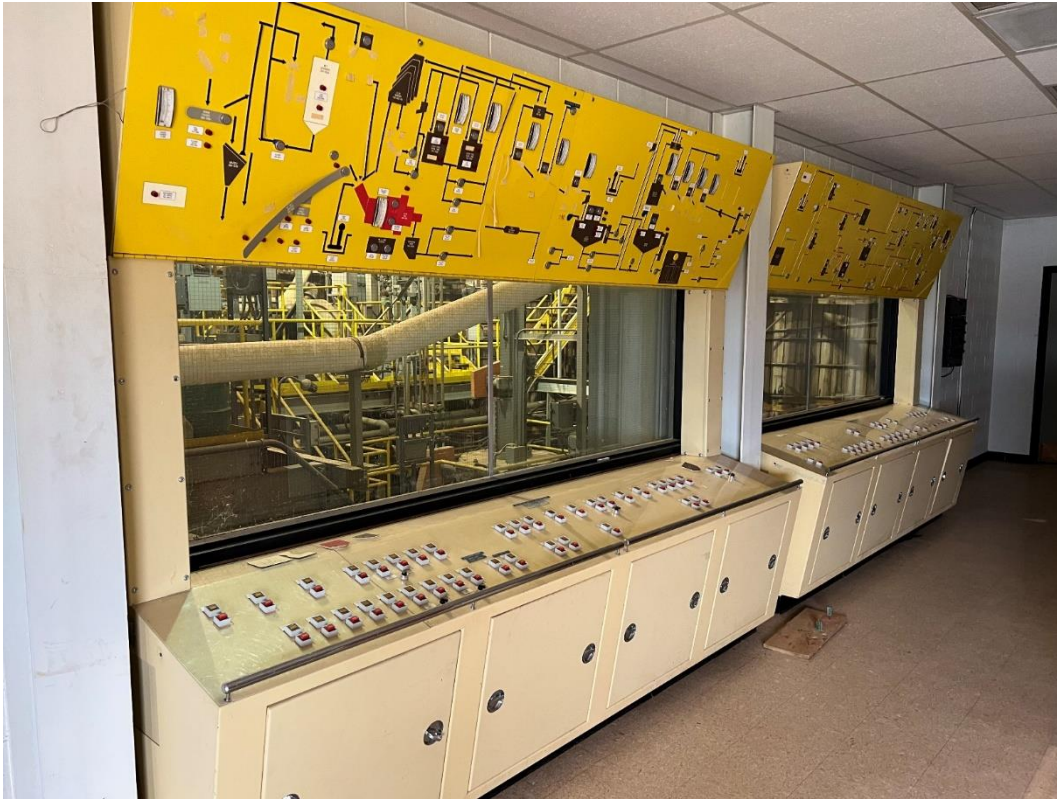
Figure 9: Upper/Lower: inside the control room at the mill – all of the systems controls will need to be modernized at refurbishment
