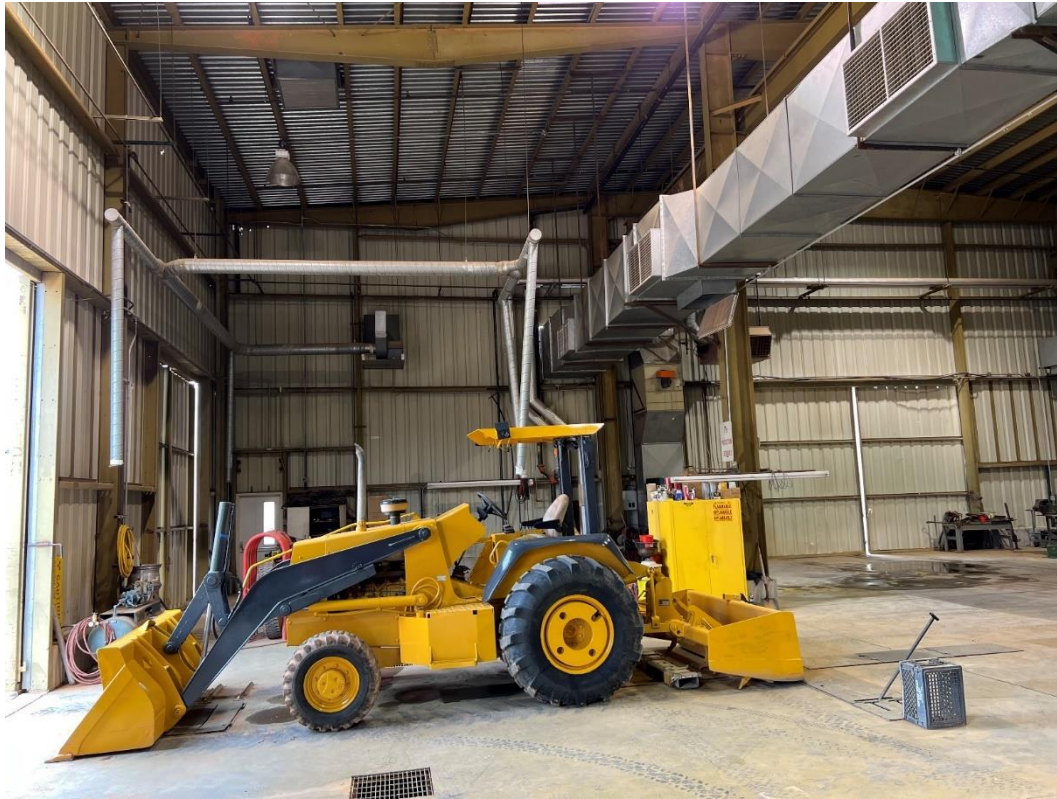
Figure 13: Upper/Lower – inside the maintenance bay at the mill – storing valuable assets (extra genset, loader)
