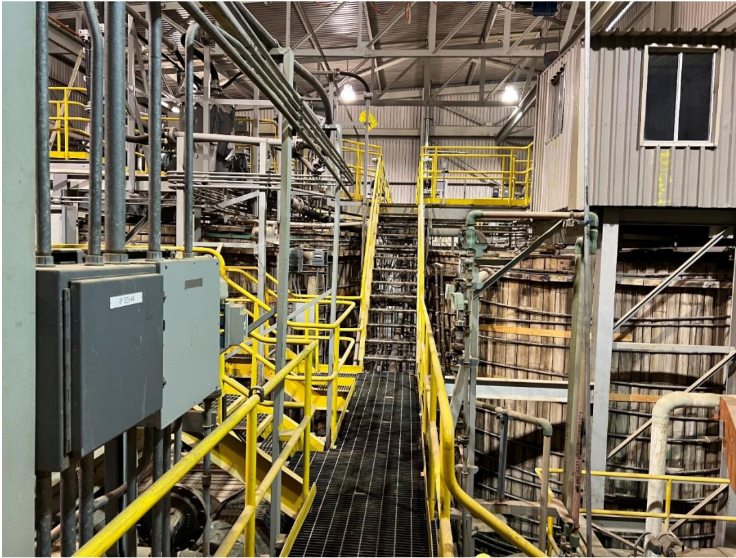
Figure 6: Supporting infrastructure for the leaching circuits (piping, air handling, valving, etc.) – all appear in very clean state of repair
