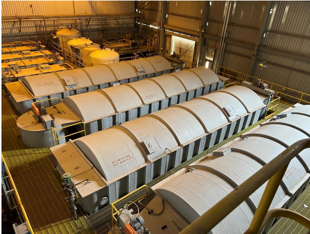
Figure 8: - Solvent extraction tanks/circuit show in very good condition – the end of this circuit is where the end-product is produced
